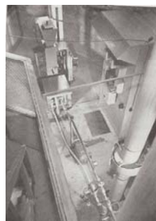
The fluoridation installation to add fluoride to the drinking water supply at the city of Tiel.
